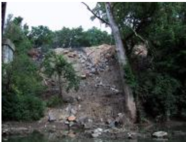
Debris dumped from Bexley's nursery on the banks of Alum Creek. Photo by David Hohmann.
